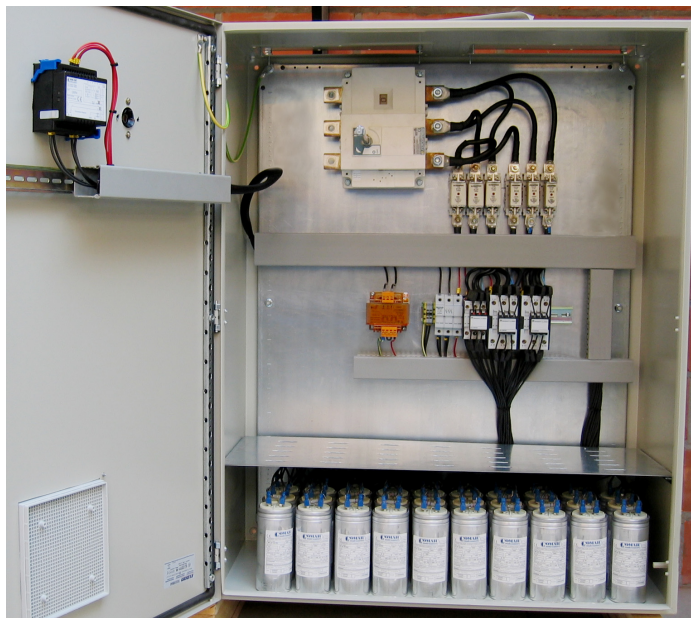
Power factor correction equipment
